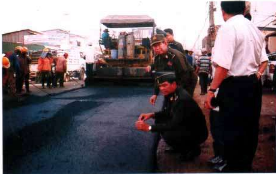
The RCAF High Command's Engineering Unit contributes actively with the Royal Government to restore and build communication systems throughout the country. HE LTGEN Kun Kim, Deputy Commander-in-Chief of the RCAF, inspects road work.
