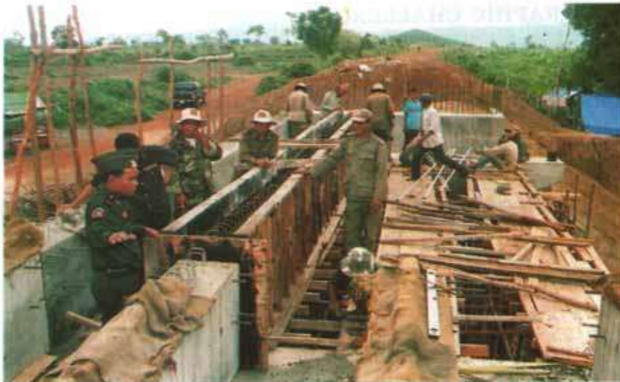
Army Engineering Forces play an important role in restoring and building physical infrastructure in remote and isolated rural areas as part of its contribution to facilitating people's livelihood.
